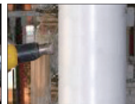
Thawing Frozen Pipes
